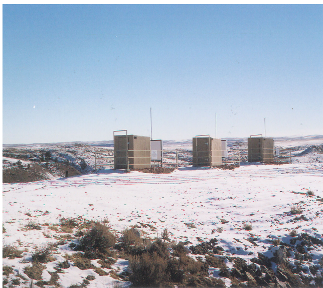
Three CBM wells finished with surface enclosures in the Powder River Basin
