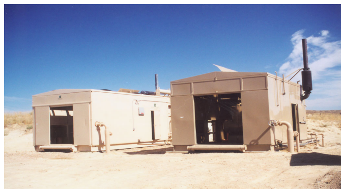
Photograph of typical CBM field compressor station
