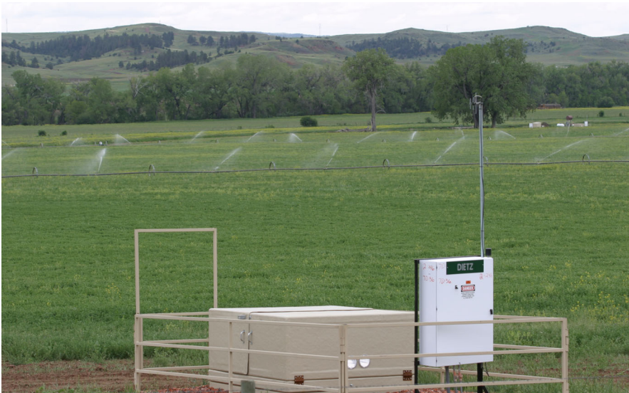
CBM well head equipped with radio monitoring system and field irrigation in background, Wyoming
